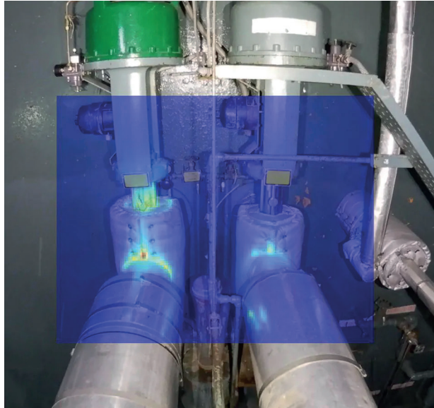
Figure 6. Thermal camera image showing a pipeline leak [11]
