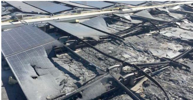
Figure 2: Roof structure damaged by solar panels
