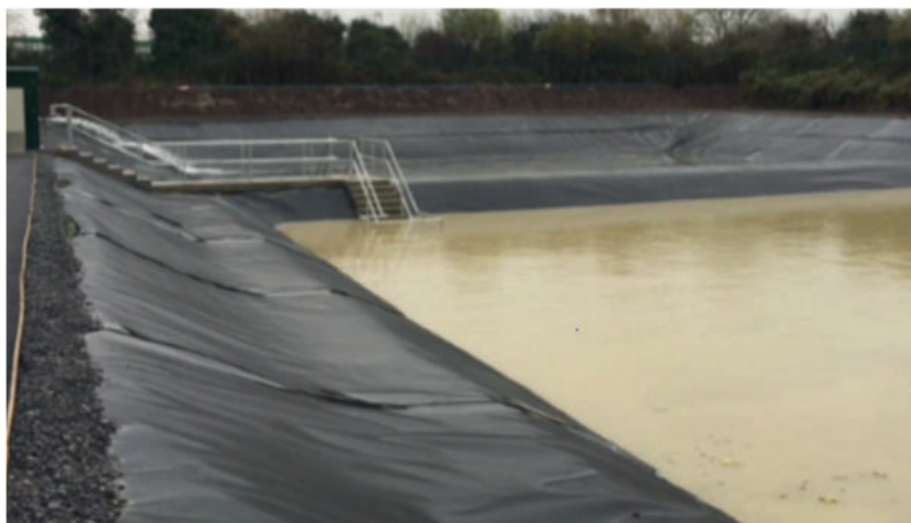
Picture 2. Fire water retention facility
