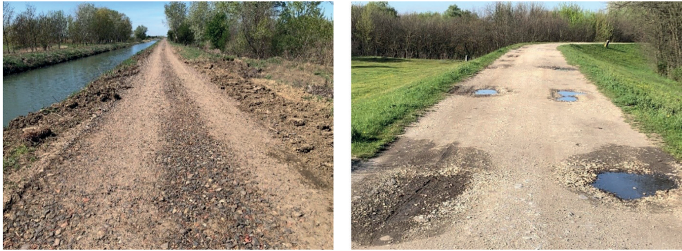
Figure 11. Gravel road in good condition and with damaged surface (periphery of Tiszasüly and Szolnok).
