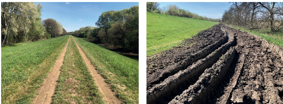
Figure 7. Well maintained and damaged unpaved road (periphery of Szolnok and Pély).
