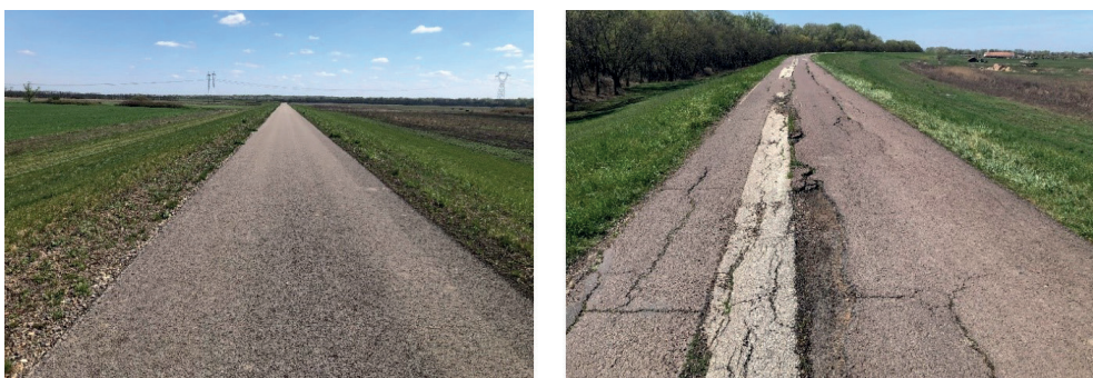
Figure 8. A tarmac road in good and damaged condition (periphery of Besenyszög and Pély)
