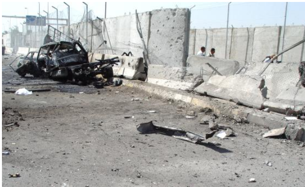
Fig. 7a: Damaged protective wall after VBIED attack
