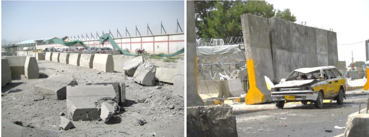
Fig. 2: Effect of VBIED on the target protective walls
