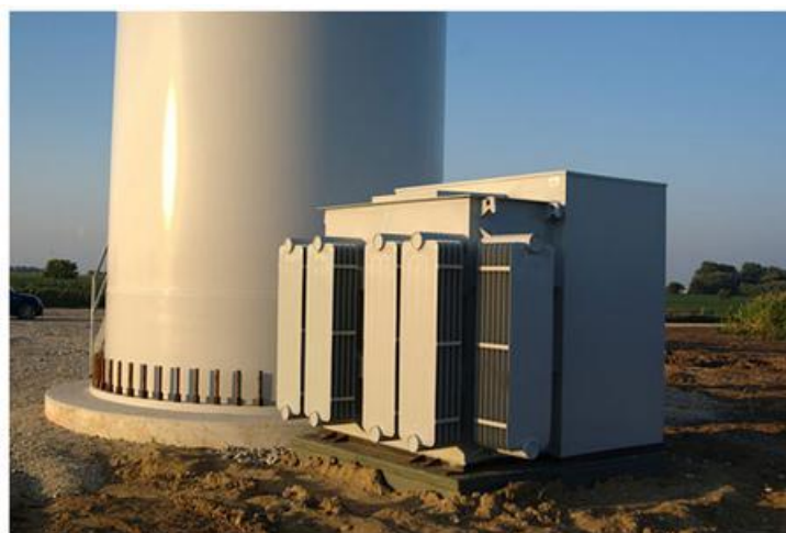
Illustration 5. Wind turbine transformer [5]
