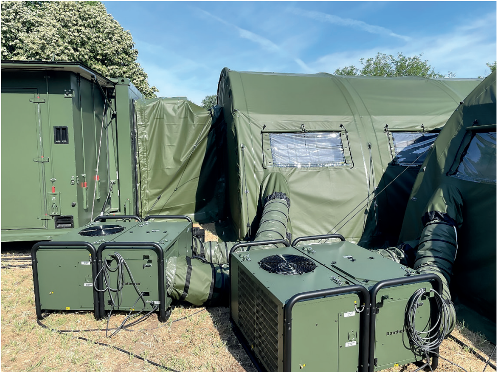
Figure 10: Container and tent interface installed, with heater-cooler unit in the foreground Source: compiled by the authors.
