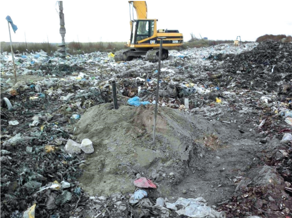
Figure 1: Finalised monitoring well (in the foreground) and one under drilling in the background Source: FAITLI–MAGYAR 2018: 5.
