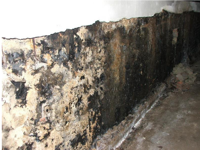
Figure 11: Tunnel lining wall incorrectly constructed (and consequently, deteriorated insulation) in a KAGRA (Kamioka Gravitational Wave Detector) facility in Budapest 13
