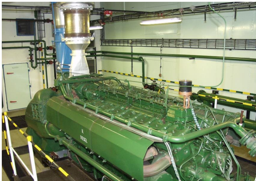
Figure 18: Power generator in the Budapest metro line [15]
