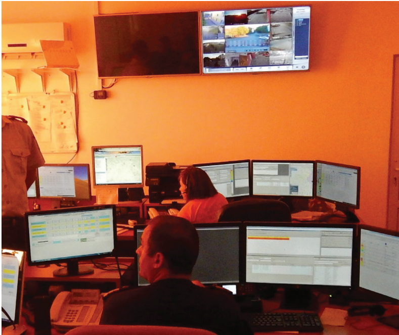
Picture 2: Dispatch unit in Romania commonly used by the fire department and the ambulance
