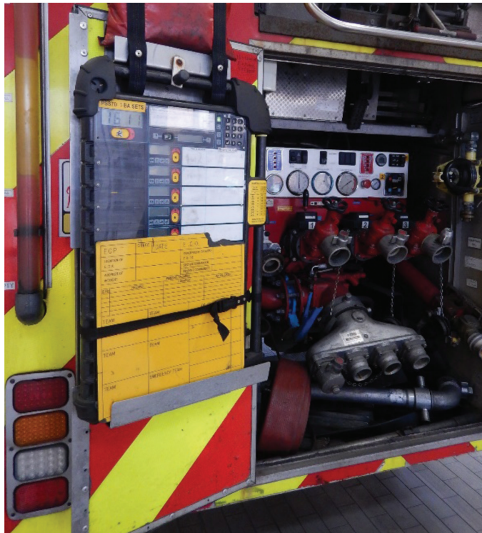
Picture 14: A Draeger Merlin system installed in a fire engine in Liverpool, United Kingdom
