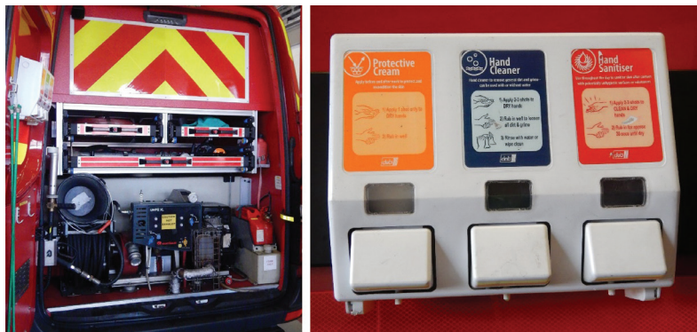
Picture 7–8: Installed hand cleaner and sanitiser unit on a fire truck in Newcastle, United Kingdom
